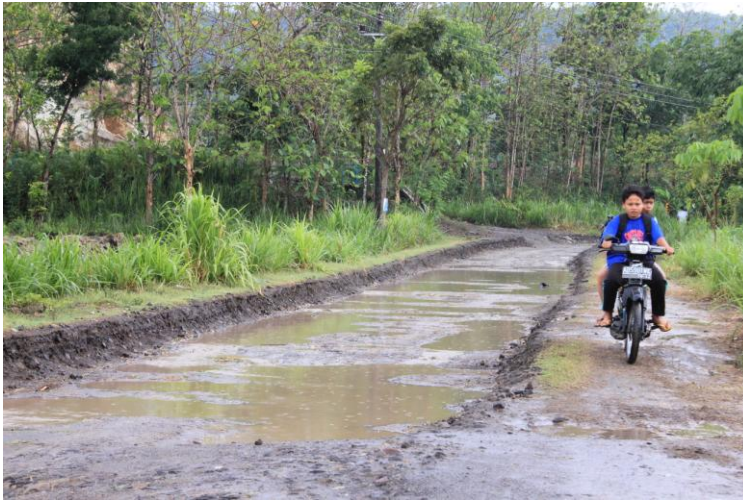
Picture 1. A slippery road heading to Wonolelo Village.
